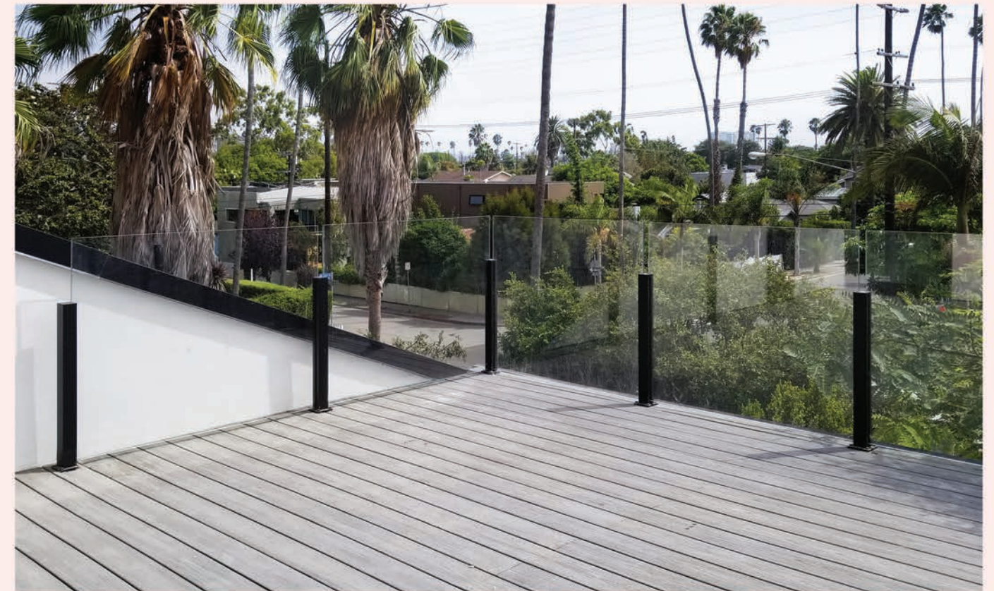
Black Painted Custom Post Guardrail
