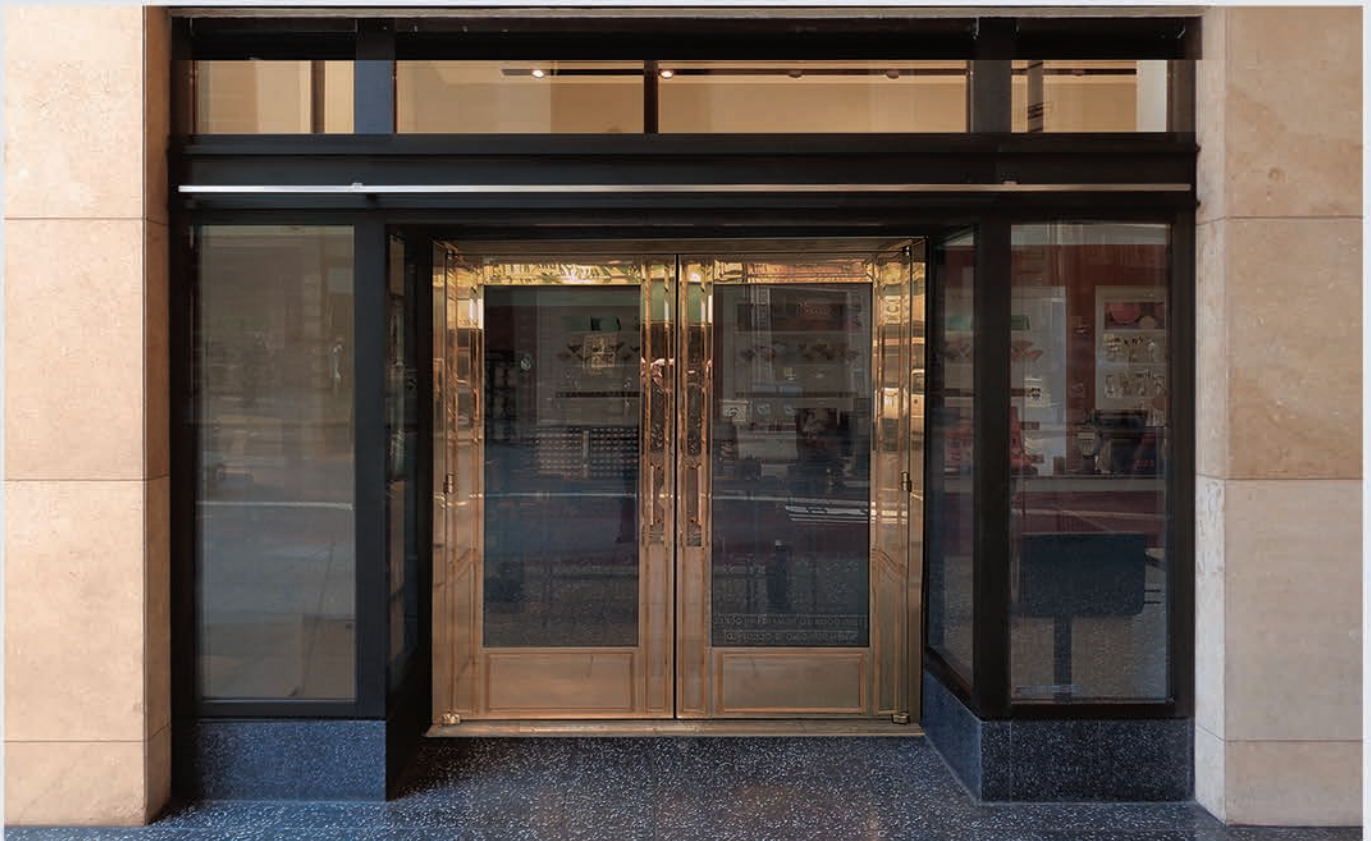
Monumental Entrance Doors with Trims in Muntz Cladded Finish and Bullet Resistant Glass
